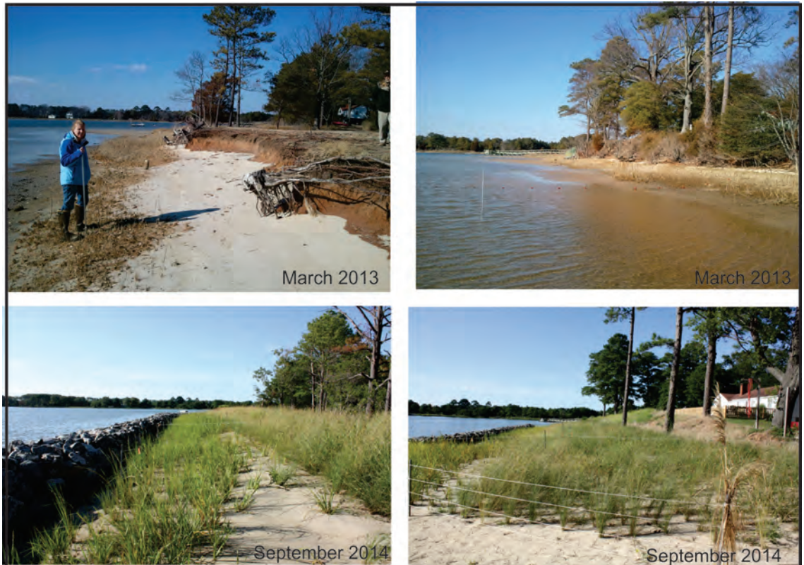
Figure 5-6. Occohannock on the Bay shoreline before (top) sill construction and after (bottom) construction.
