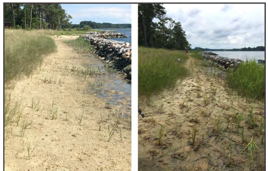
Figure 5-8. Photos showing a bare spot behind the sill (left) in May 2017, and the grasses replanted in July 2017 (right).
